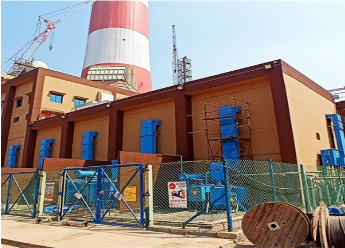
Electrical & Control Building
