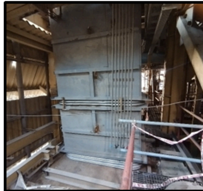
SOFA Duct taken from SA Duct
