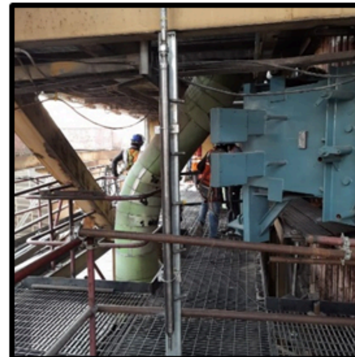
Instrument air header at corner 4 for SOFA operation
